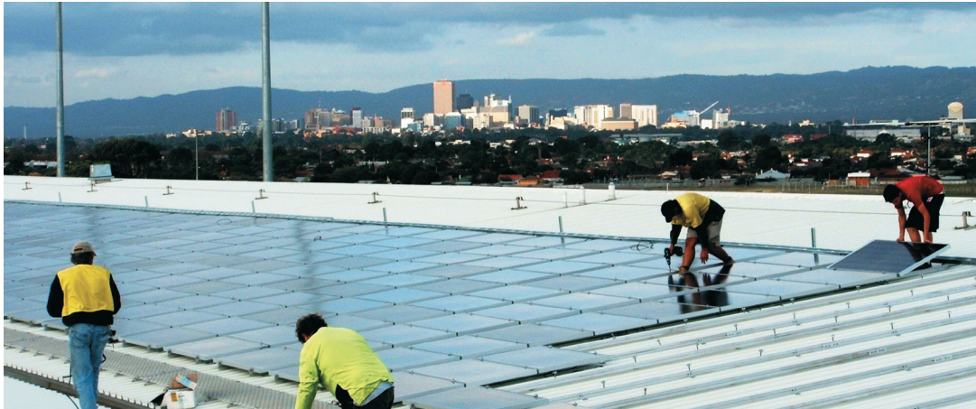
Adelaide Airport's grid-connected rooftop solar installation (Photo courtesy of Adelaide Airport)
