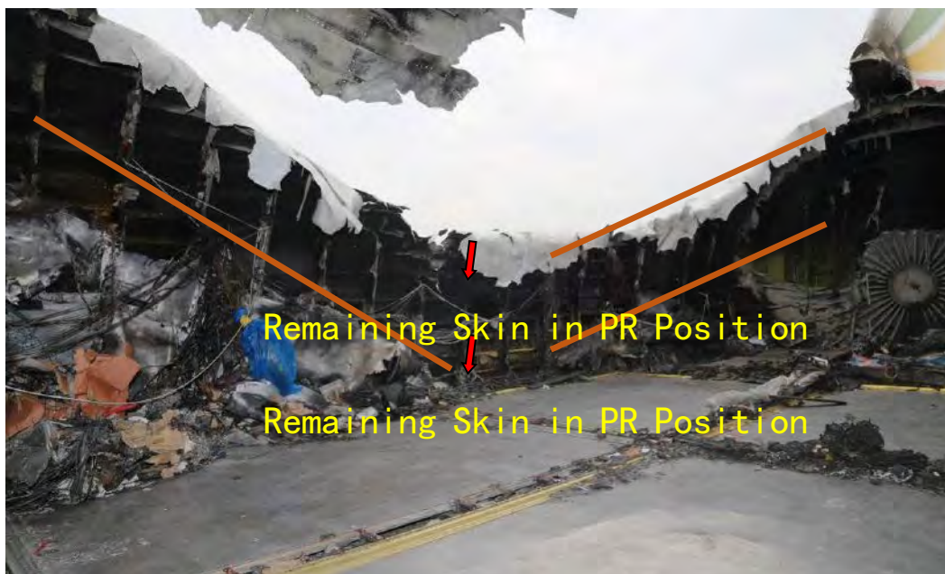
Figure 66 Remained Skin and Frames at PR Position (Interior View)
